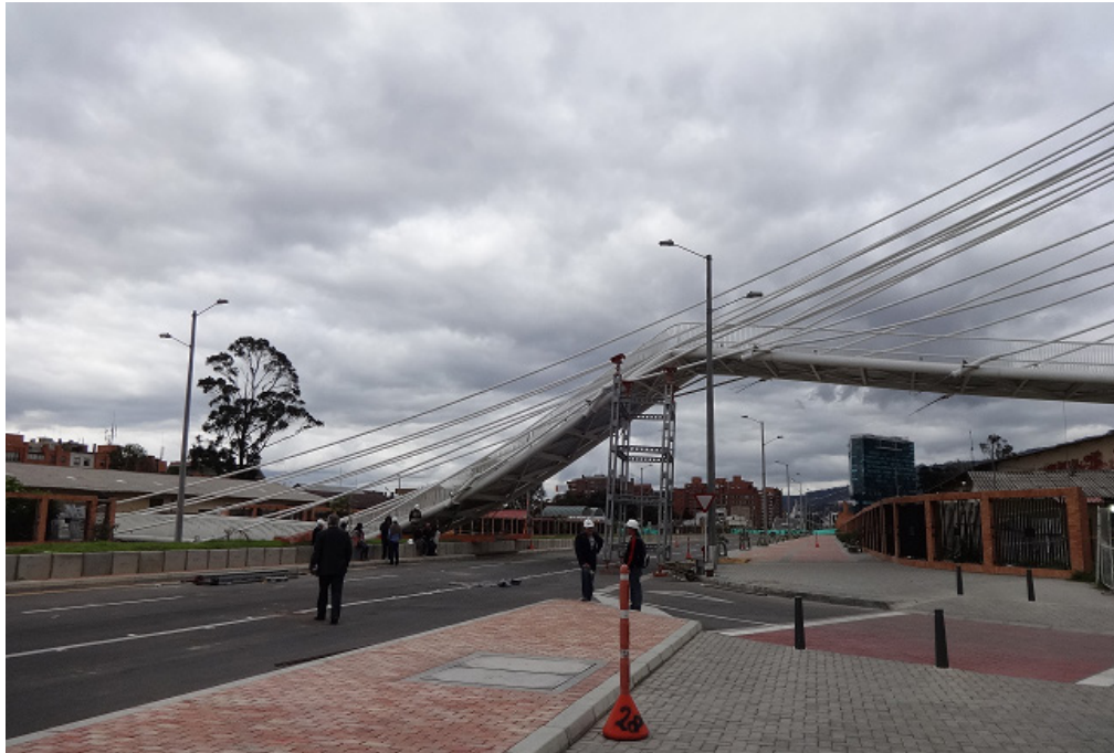
Photo 1. Failure of Cantón Norte Bridge. Source: Photo by Zulma S. Pardo V.
