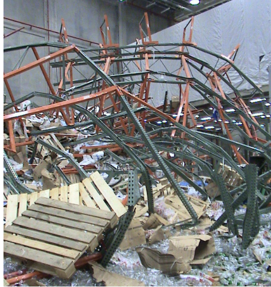
Photo 2. Failure a rack structure. Source: Photo by Zulma S. Pardo V.
